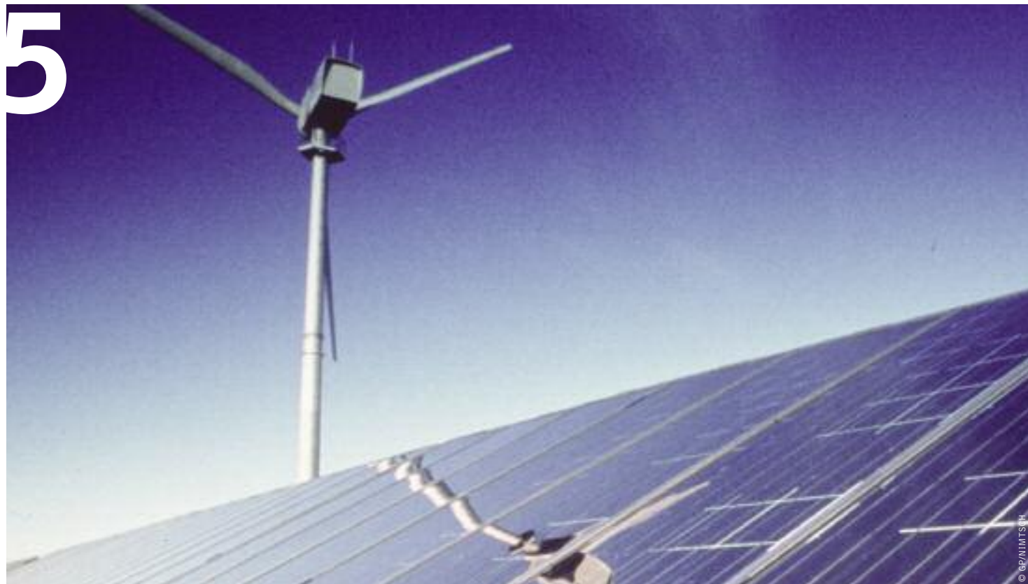
image SOLAR AND WIND-FACILITY NEAR ROSTOCK, GERMANY.
