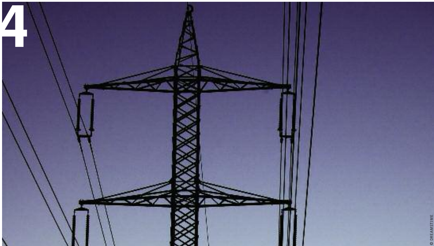
image ELECTRICITY LINES.
