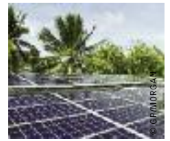
image SOLAR PANELS ON REFRIGERATION PLANT (FOR KEEPING FISH FRESH). LIKIEP ATOLL, MARSHALL ISLANDS.
